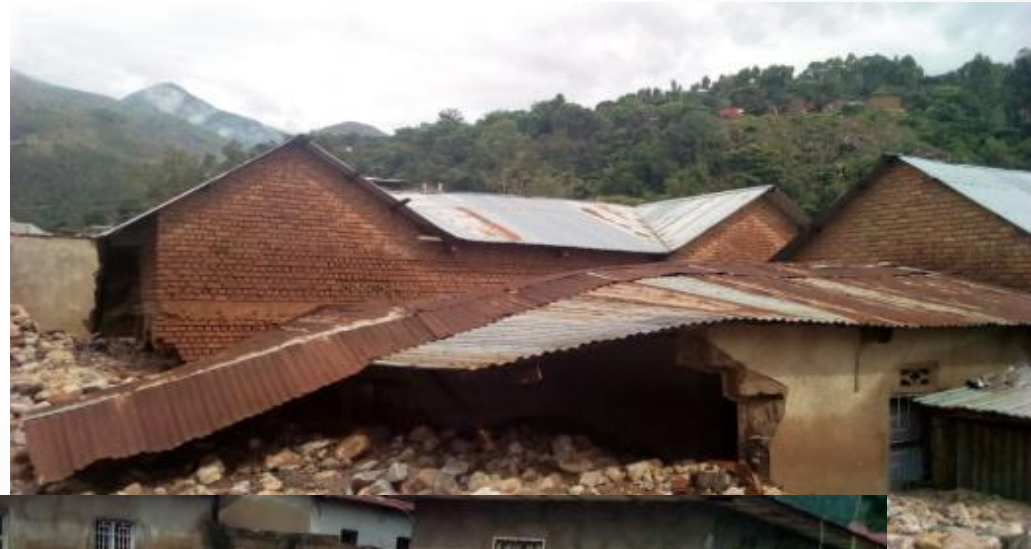
Flood damage in DRC, Rwanda, Burundi
