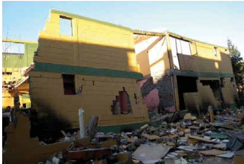
Image 2: A building with a collapsed ground floor as a result of the February 2010 earthquake in Chile. Source: Brzev, Astroza and Yadlin, 2010 22 .
