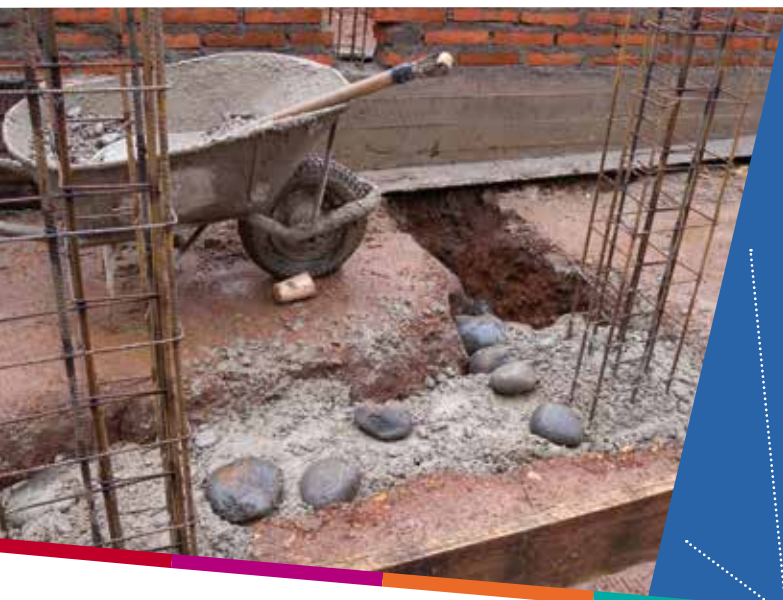
Image 1: Tie-column reinforcement cages extending from foundations of a new building; these are a key feature of 'confined masonry' construction. Source: Brzev, Astroza and Yadlin, 2010 1 .
